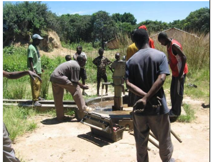
The repairs are completed and clean water is available to the community.
