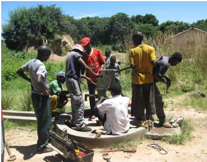
Young men from the community assisted the Seeds of Hope Pump Repair crew.
