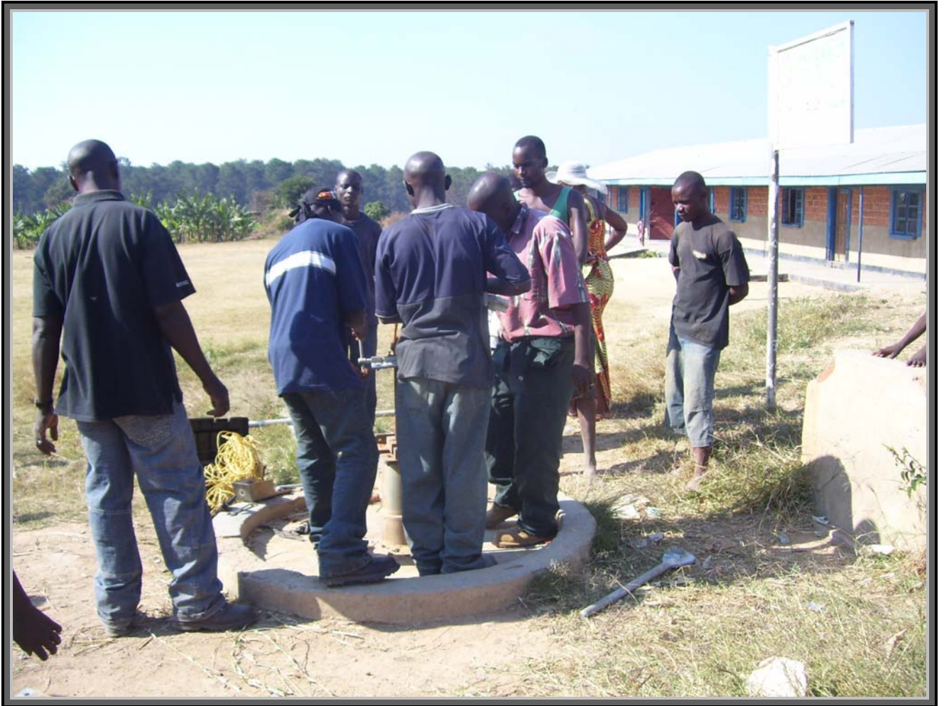
This is a pump repair in Kawama, at Community Institute for development
