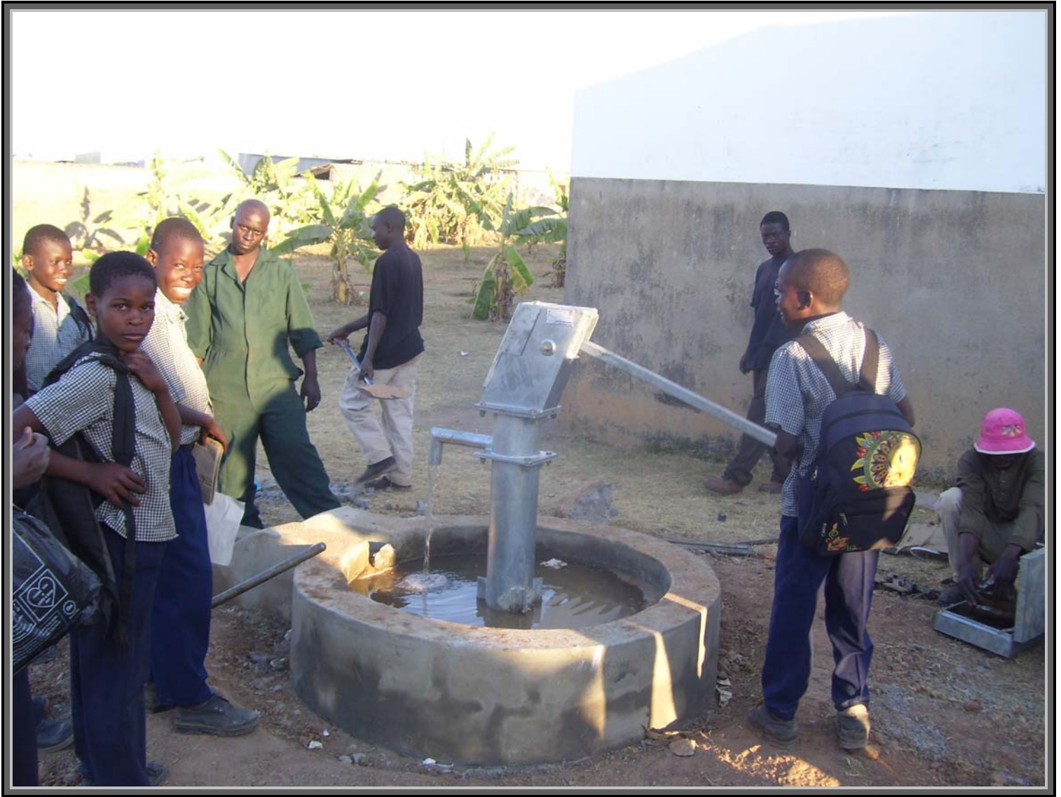
Here goes the newly installed pump; we have water for the school.
